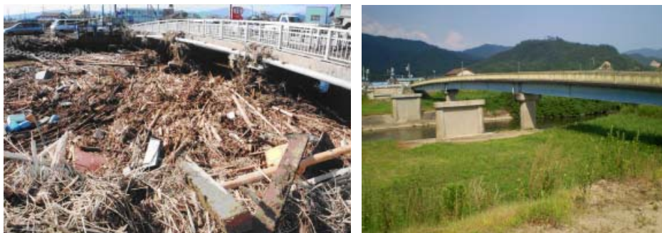
Photos showing floating debris from nearby mountains and forests that blocked rivers and damaged bridges on the left, and well maintained rivers and embankments on the right.
