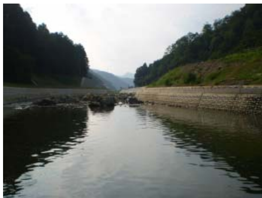
The Maruyama river today, with its strengthened embankments that is also a place of attraction for local residents to relax.
